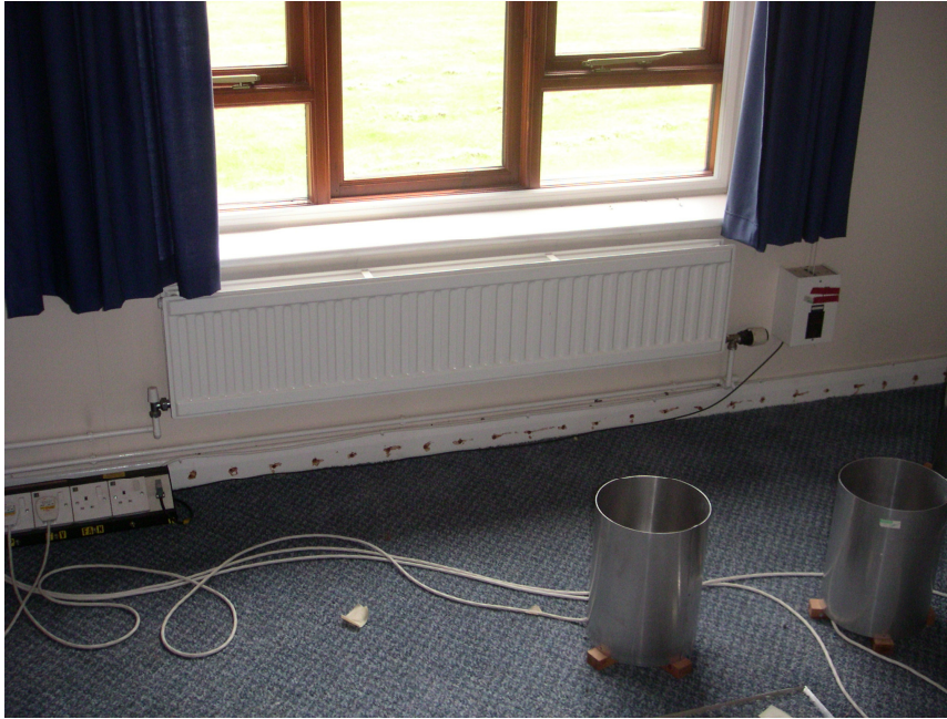
Figure 36 Visual picture of the traditional steel panel radiator in the lounge of House 1
