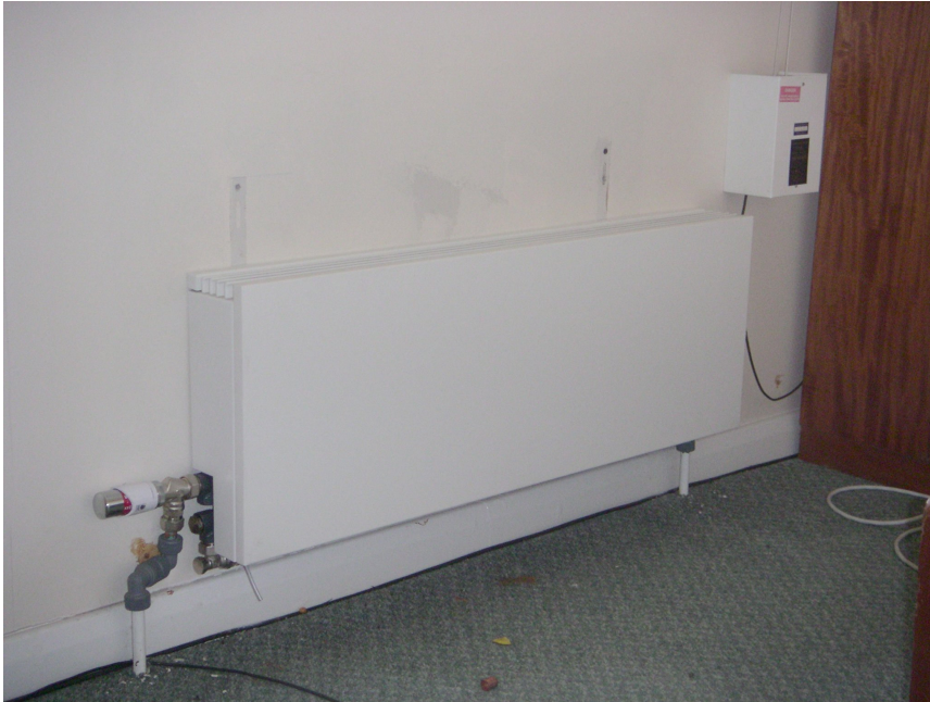
Figure 27 Visual picture of the Jaga low H 2 O heat emitter in Bedroom 1 of House 2
