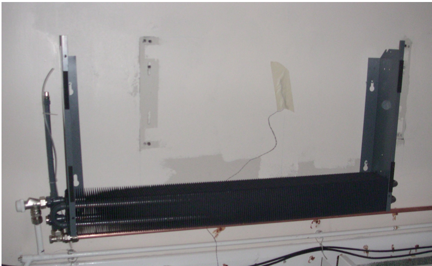
Figure 28 A Jaga low H 2 O emitter with casing removed (note the thermocouple affixed to the wall recording surface temperature).
